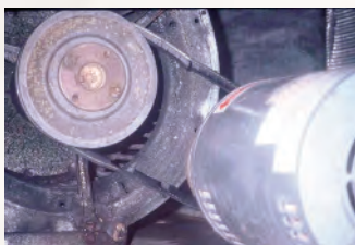
Fan belts should be checked regularly and replaced as necessary – this belt is not fit for use.
