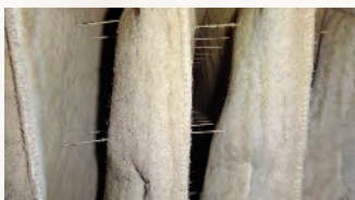
Air filters need to be checked and replaced regularly
