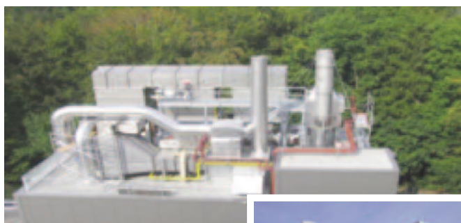
The Erbo Spraytec facility in Switzerland.
