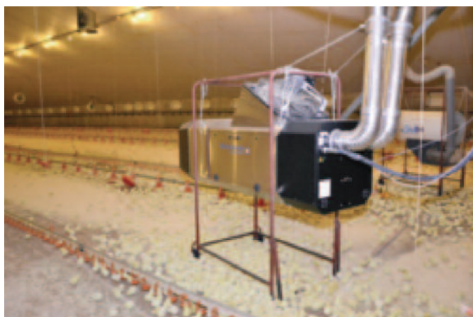
Indirect fired unit, Winterwarm DXC heater.
