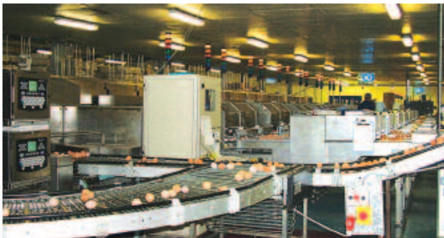
Part of the busy in line egg packing plant with graders linked directly to Flockdata via fibre optic cables.
