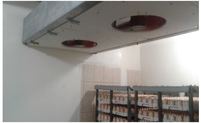
A room fitted with an overhead fan and heating elements can also be a good option to utilise as a pre-warming chamber.
