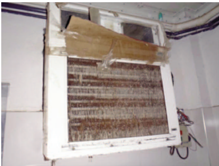
An example of an air conditioning unit in the egg room that has not been properly maintained.
