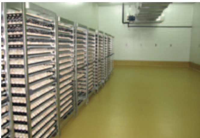
Left, the egg store and, right, inside the setter room with the SmartPro Setters. Above right, the corridor between the setter rooms.
