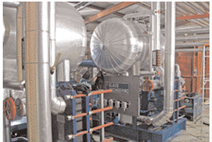
The air treatment equipment.
