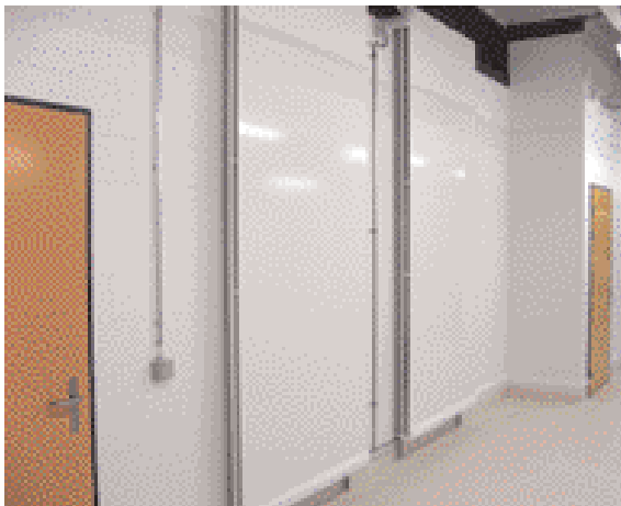
Special radiators maintain air temperature in the transfer room.
