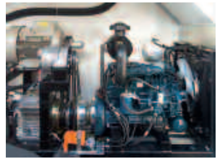
The diesel engine and electromotor with the compressor.
