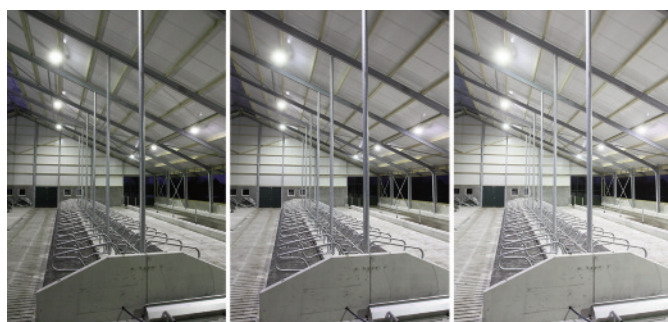
LED high bays dimmed to 30W on left and at full 150W on right.
