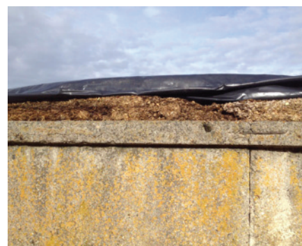
Poor sealing with ongoing air stress.
